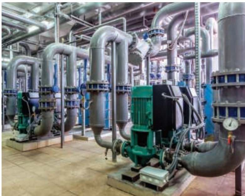
FIGURE 6. Centrifugal pump failures are often caused by pump users attempting to operate pumps in parallel without the proper equipment review, procedural review or instrumentation
