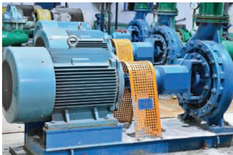
FIGURE 1. When parallel pumps are installed and operated in parallel, individual pump flows are additive, but pump heads are not. Problems often arise when operators assume the pumps are identical in head and flow characteristics and that flows will remain similar throughout the pumps' lifetimes
