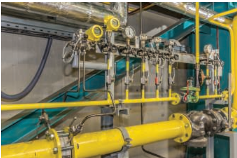
FIGURE 2. This photo shows flow measurement via an orifice plate and mechanical DP measurement. The static pressure is measured by an additional sensor
